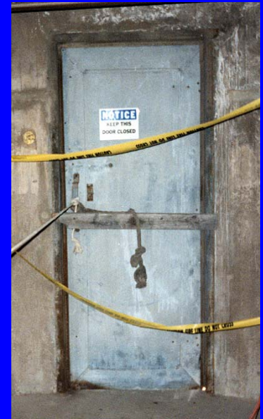
Locked and blocked exit
